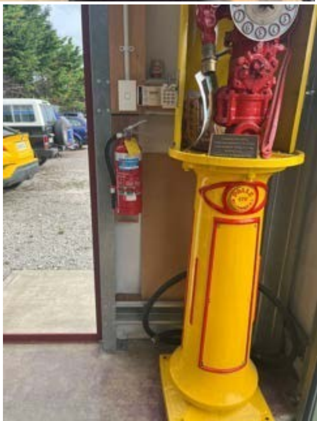
Photo of the re sited extinguisher, please familiarise yourself with it's new location
