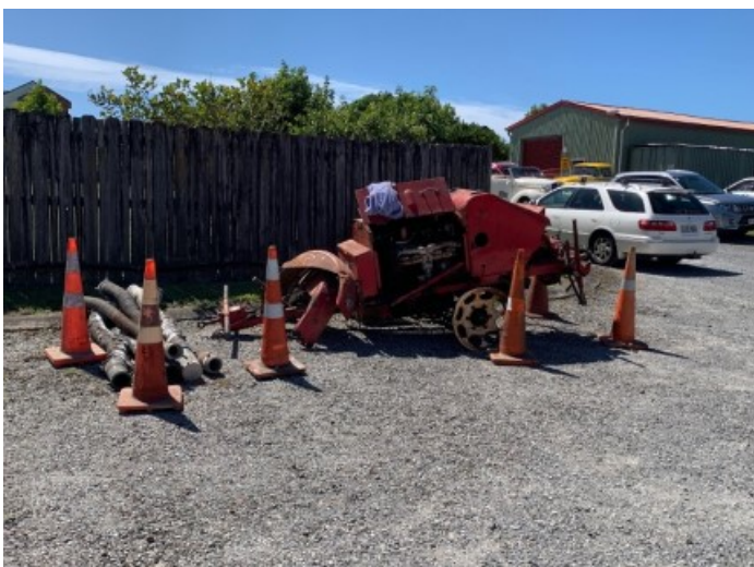
The Fire Pump in the yard ready for collection.
